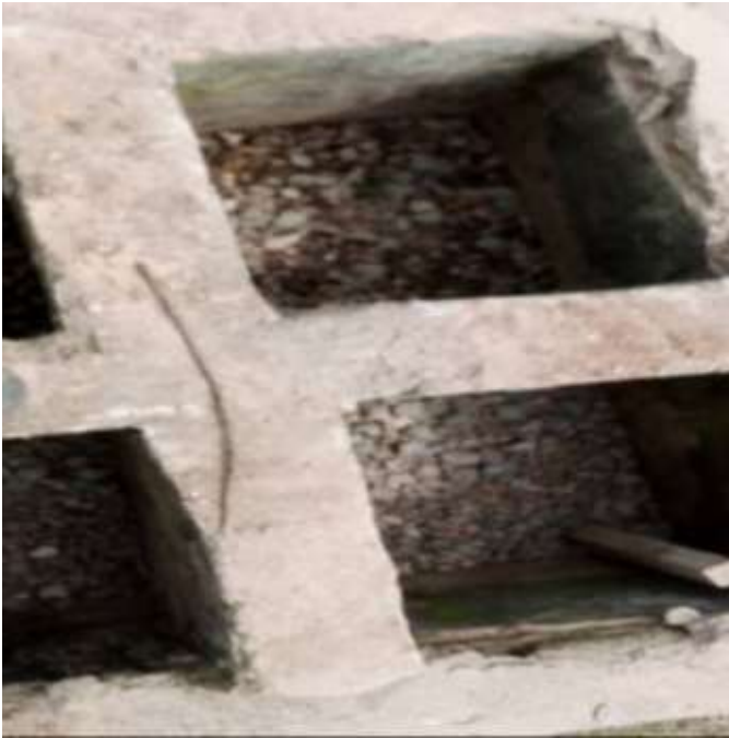
Figure 21: Layer of aggregates in filter media
