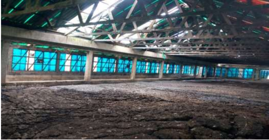
Figure 9: Sedimentation /thickening tank at Lubigi waste water Treatment Plant.
