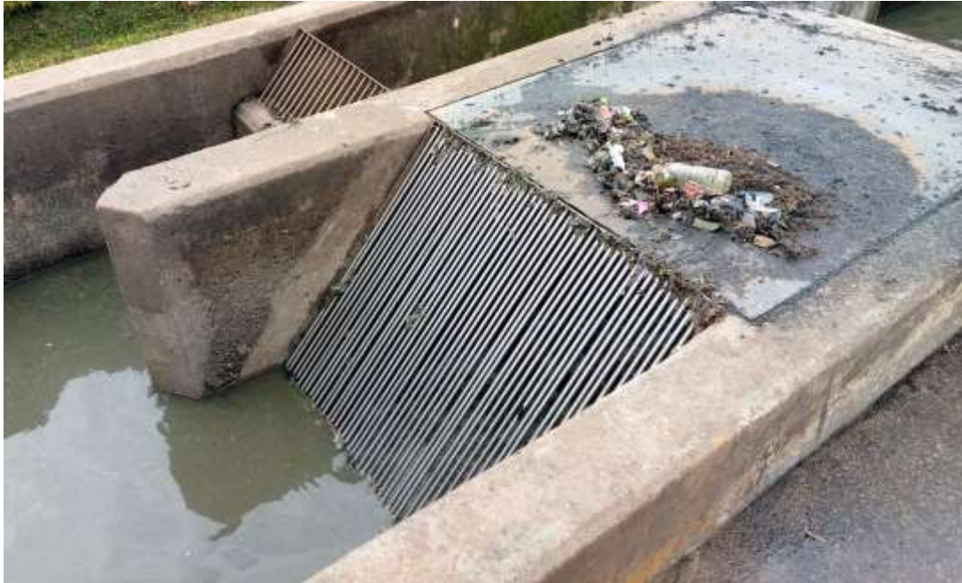
Figure 8: Screening process at primary stage of treatment.
