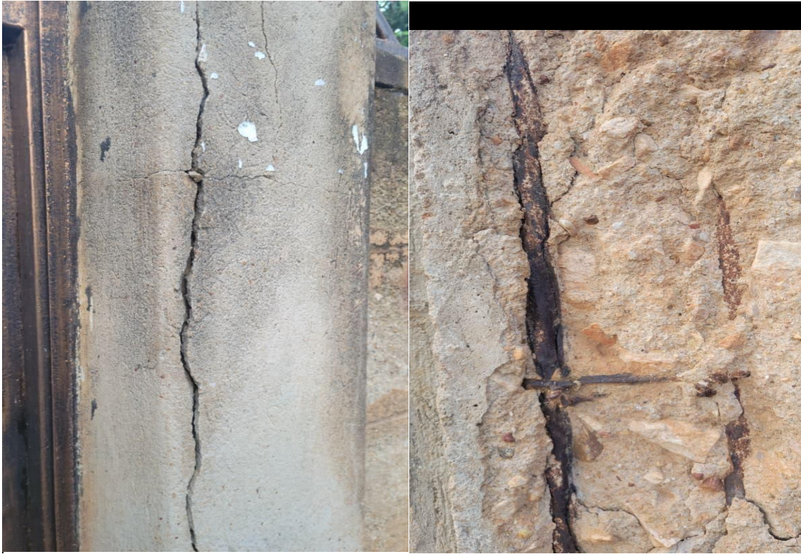
Figure 1: Images showing the start of spalling in a reinforced concrete column(left) and a column with lost concrete cover (right) at CNN hostel.
