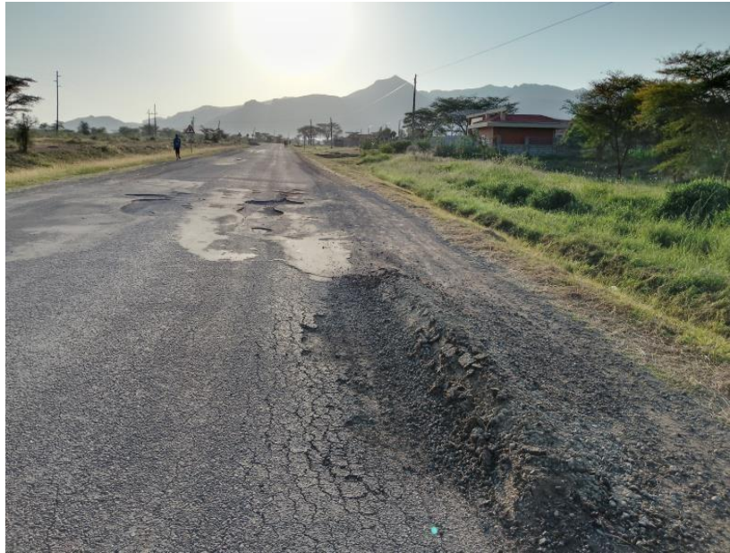
Figure 2 Pavement failure of one or the road sections of the Soroti Moroto road taken during one of the site visits.
