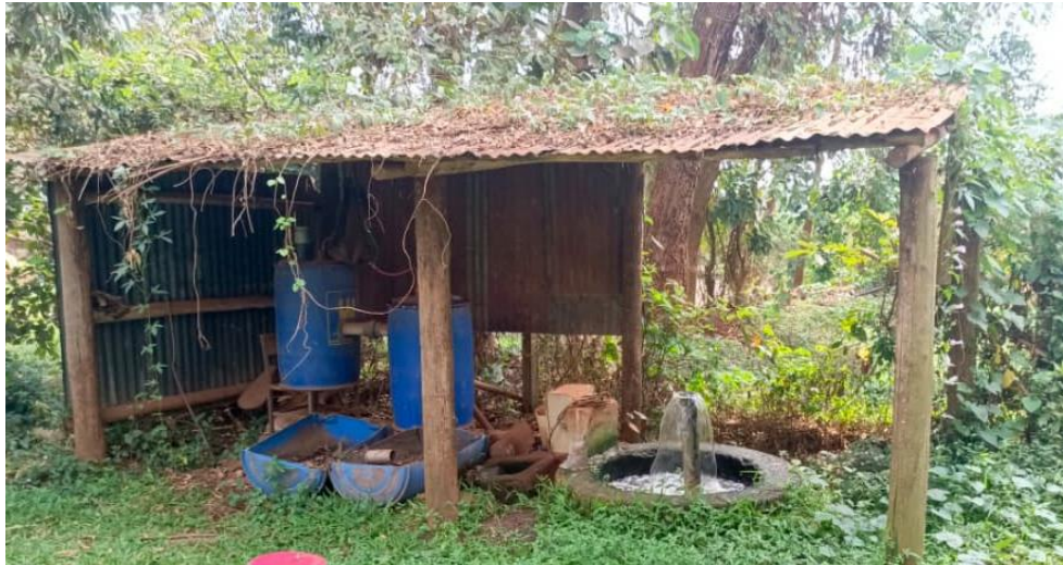
Figure 28: The UCU activated sludge treatment plant effluent discharge point.
