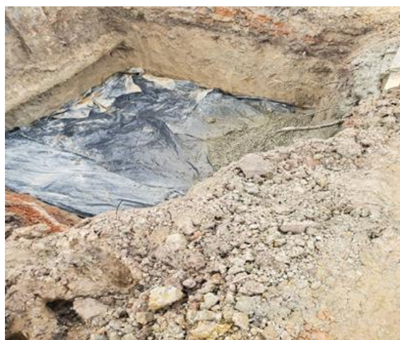
Figure 1: Silty clay soils foundation challenges.
