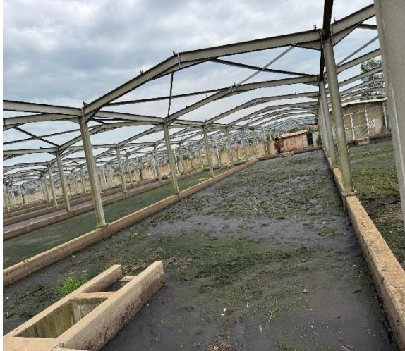
Figure 6 Sludge drying beds
