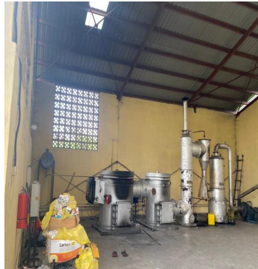
A typical mass-burn incinerator
