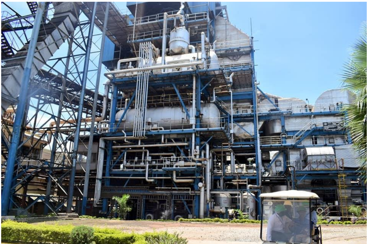
Figure 3: Kakira's bagasse cogeneration power plant
