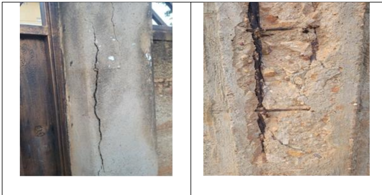
Figure 1 Images showing the start of spalling in a reinforced concrete column(left) and a column with lost concrete cover (right)
