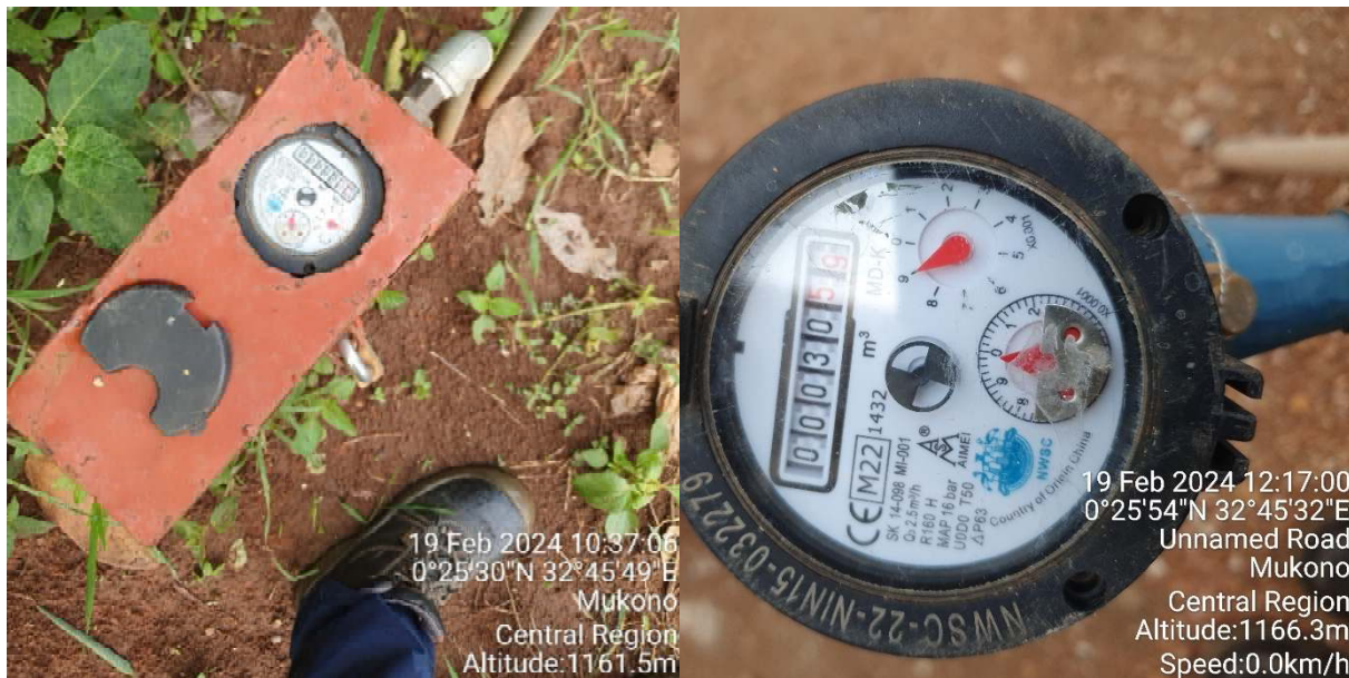
Figure 19: Images showing some of the customer meters.
