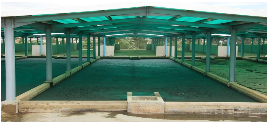
Figure 3: Settling /thickening tank at Lubigi Treatment Plant (Nabaggala, 2023).
