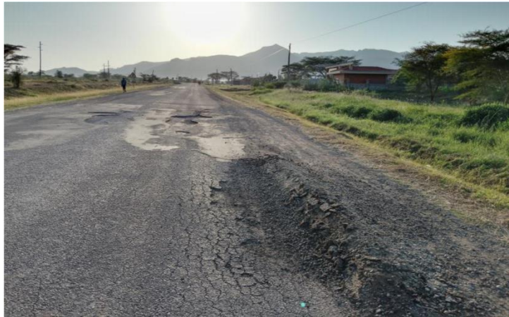
Figure 2: pavement failure of one or the road sections of the Soroti Moroto road taken during one of the site visits
