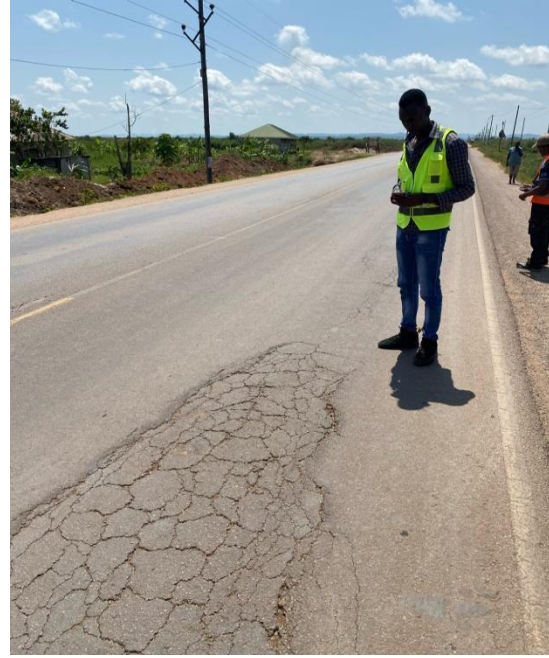
appendix 2 Site visit to the failed section
