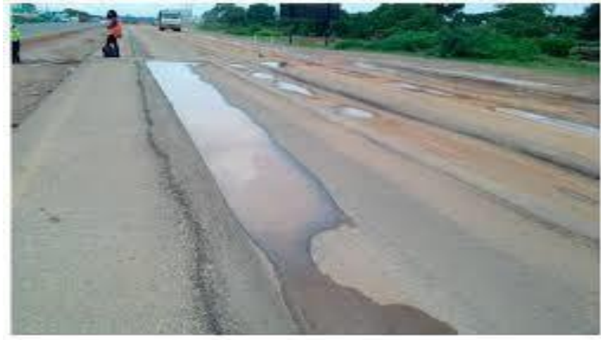
Figure 2:2 Rutting on an asphalt pavement (Handbook of Highway Engineering, 2024)
