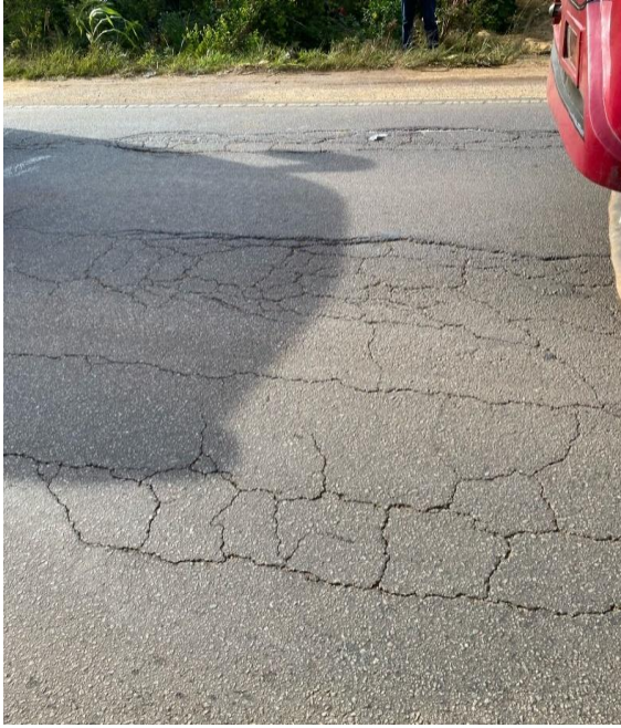
appendix 1 Failed section along the highway
