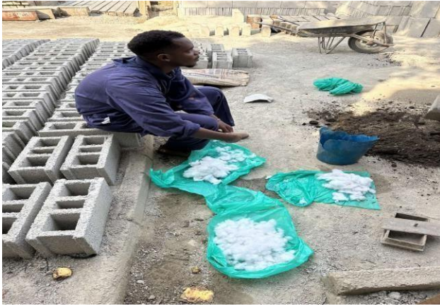
Figure 11:APPLICATION OF REPRESENTATIVE FRACTION OF PRE SOAKED FIBER ON THE CONCRETE MIX BEFORE CASTING
