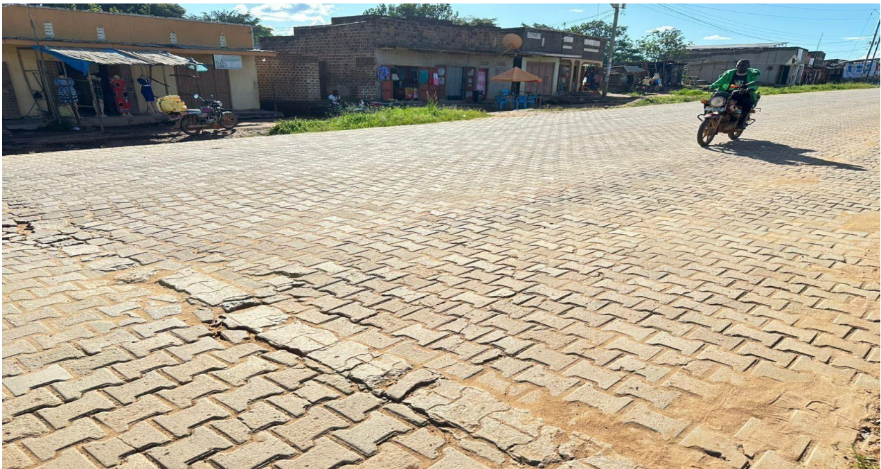
Figure 1: showing a section of the cracked pavers at kanyanda town along matuuga kapeeka road
