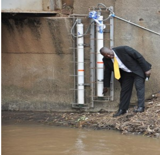
Figure 5.2: Water Level Sensors by Namulo bridge to detect water levels in Butaleja district.
